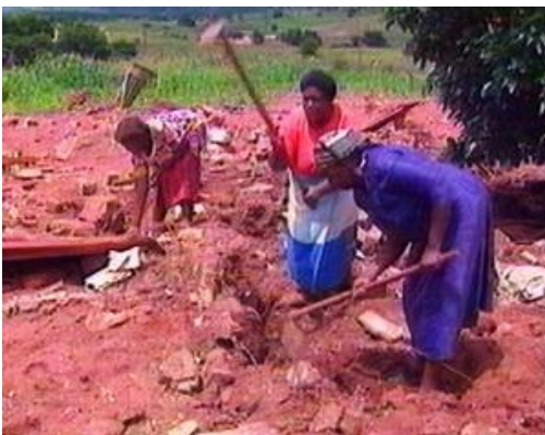
Image 7 - Clearing the rubble: The image above shows Pedi women using rudimentary tools to clear rubble from a low level bridge in Limpopo Province. The text of the image indicates that the bridge had been destroyed by heavy rains about five months before
